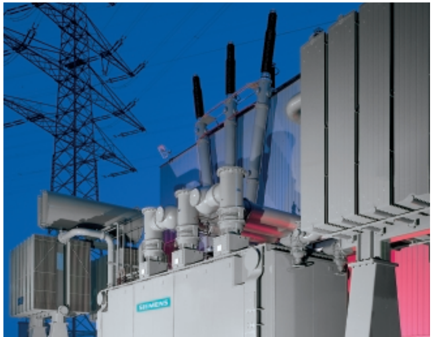
Fig. 15: Direct SF 6 -connection of the transformer to the switchgear
