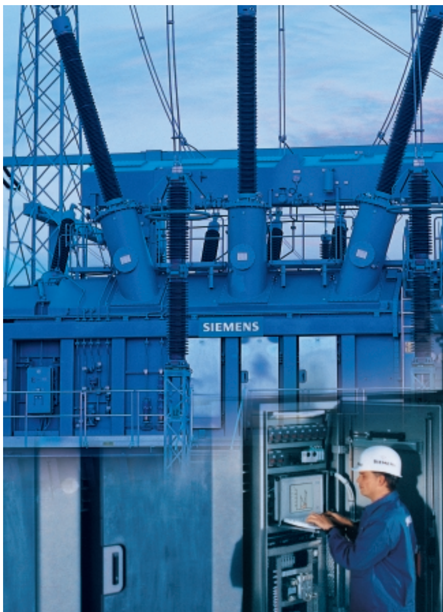
Fig. 45: An integrated solution – the complete Monitoring System housed in a cubicle of the transformer itself
